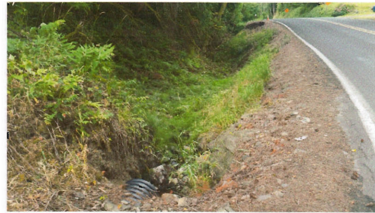
TAKEN NEAR THE 12" CPP ON THE SOUTH SIDE OF THE INTERSECTION AT THE NORTHEAST END OF THE PROJECT, LOOKING SOUTHWEST, TOWARDS THE SLIDE
