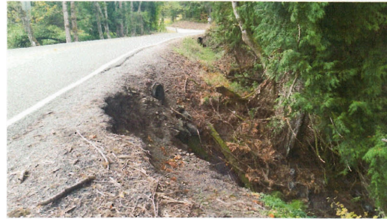
TAKEN ON SOUTHEAST SIDE OF ROAD, LOOKING NORTHEAST TOWARDS SLIDE AREA
